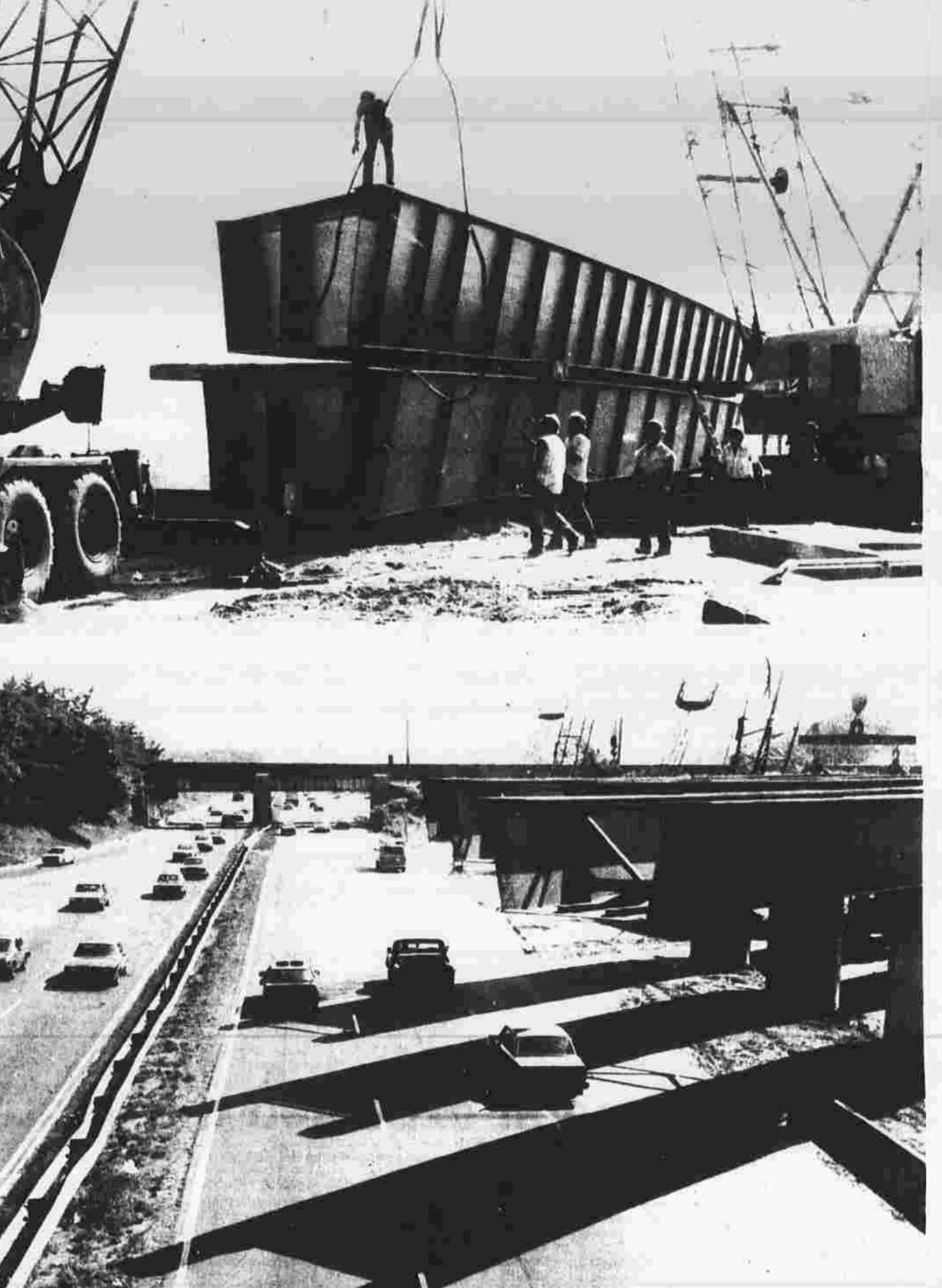
Overpass is growing. The two massive girders which construction workers are hoisting to a crane in the top photo became part of the new Toland Turnpike overpass above I-86 minutes later on Thursday, spanning across the section of highway seen in the photo above.
